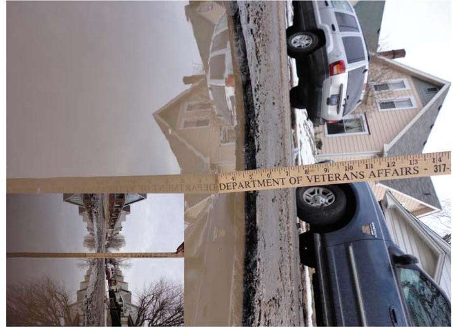
▲ Multiple Instances of Potholes Greater than 3.5" Deep
