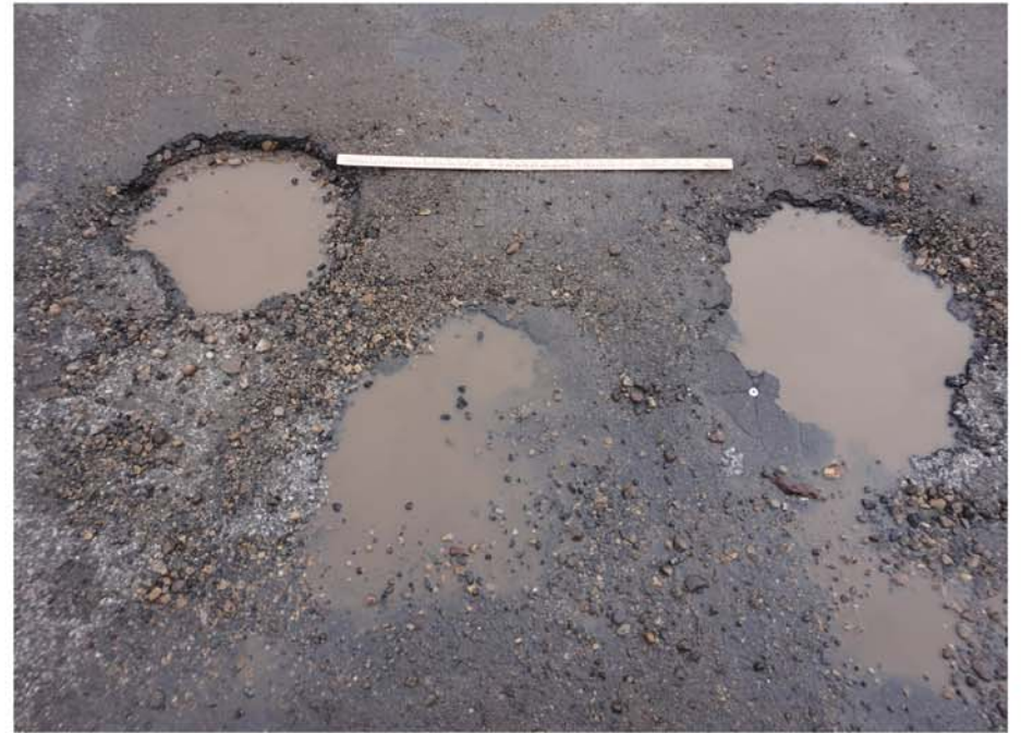
▲ Yard Stick by Potholes & Loose Aggregate
