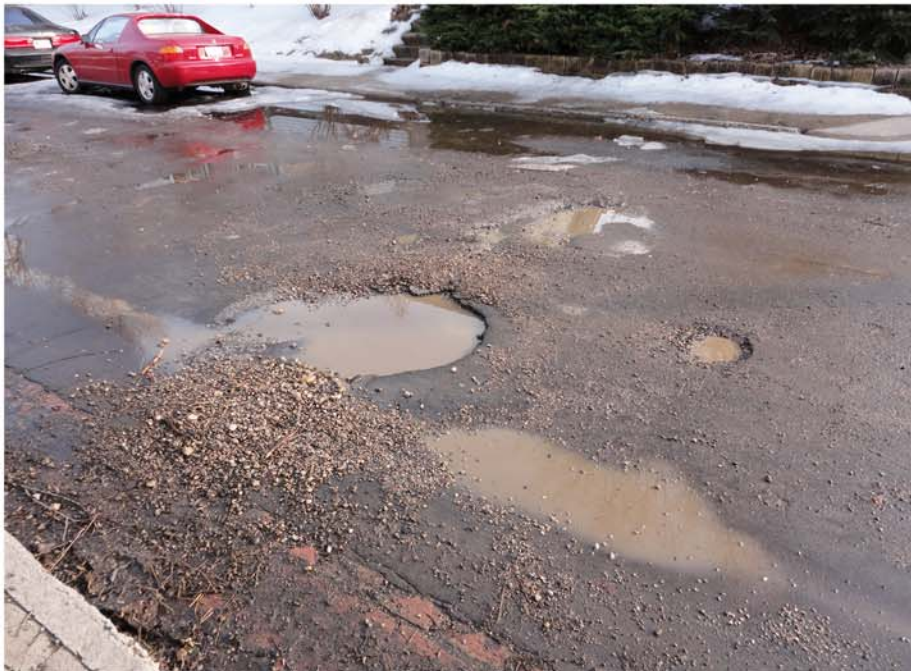
▼ Potholes & Loose Aggregate, 700 Block of Orange
