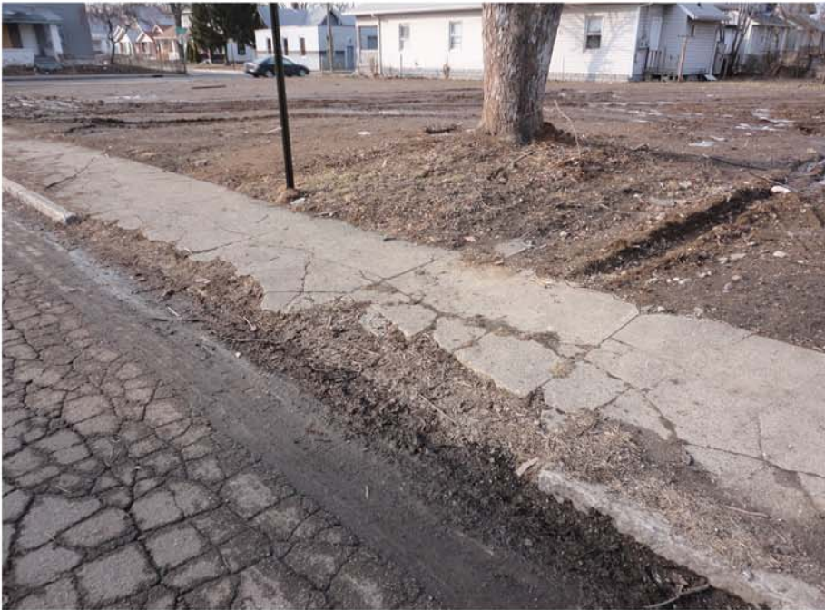
▲ Severely Deteriorated Curb, 500 Block of Orange
