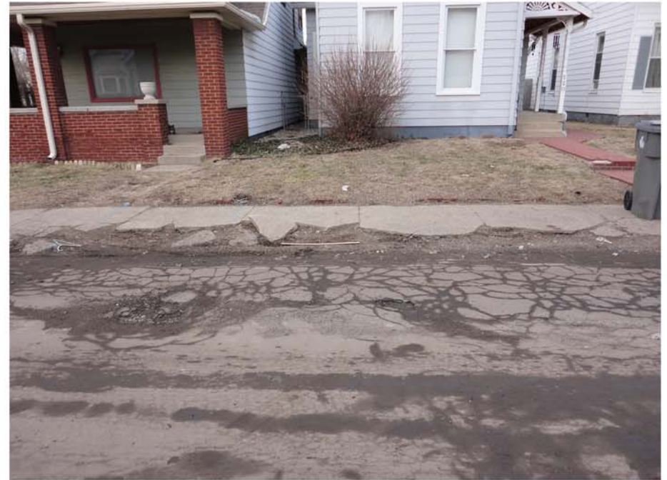
▲ Yard Stick alongside 20+ Foot Stretch of Broken Walk, 500 Block of Orange Street
