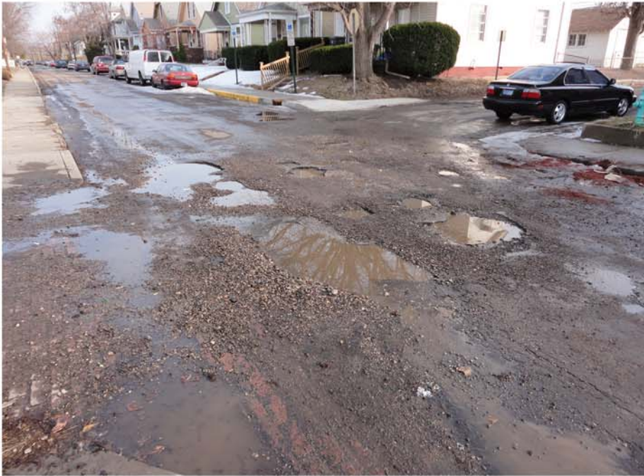
▲ Potholes & Loose Aggregate, Orange St & Elmwood Ave
