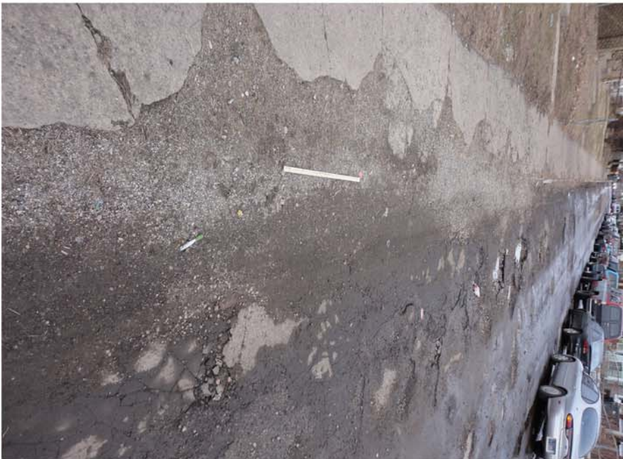
▼ Yard Stick alongside 20+ Foot Stretch of missing walk, 600 Block of Orange
