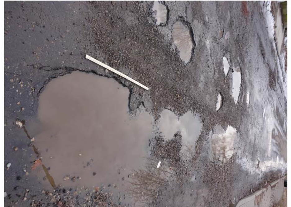
▼ Yard Stick alongside Potholes, 600 Block of Orange
