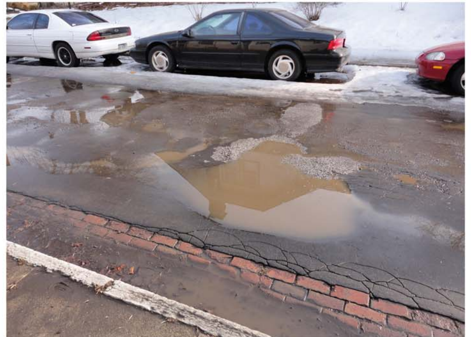
▼ Potholes, 700 Block of Orange
