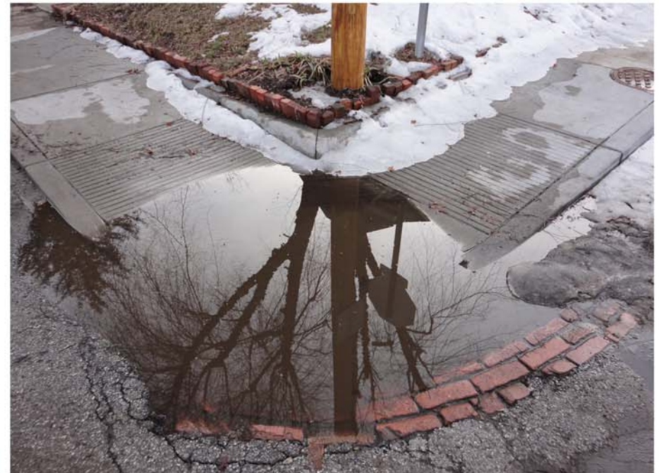
▼ Pooling Water at Wheelchair Ramp, SW Corner of Orange St & Wright St
