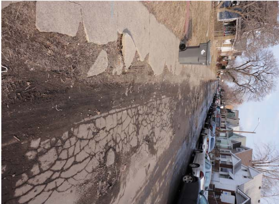
▼ Severely Deteriorated Sidewalk & Paving, 600 Block of Orange
